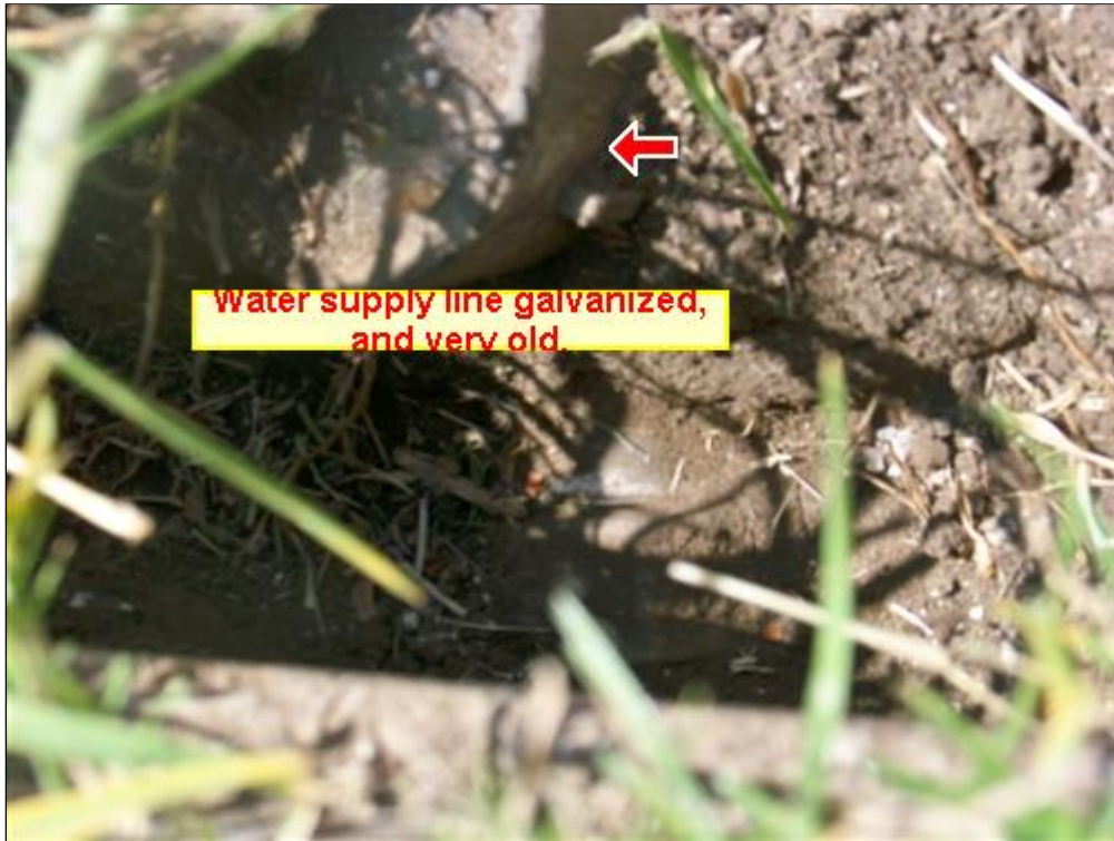
4.1 Picture 1 Water Supply at the Curb
